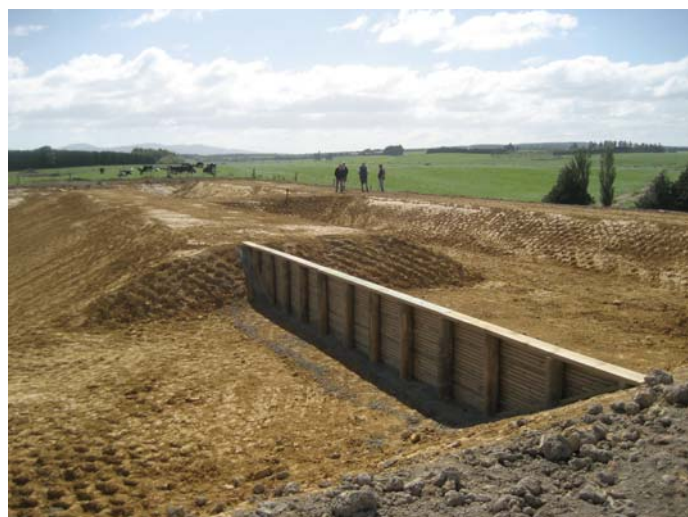
The effluent storage pond under construction at Hedgehope Pastoral (Southland) in March. The pond is 70m long, 45m wide and 4m deep with 2 liners to prevent leakage. The new design separates solid and liquid waste and has a 60 day holding capacity.
