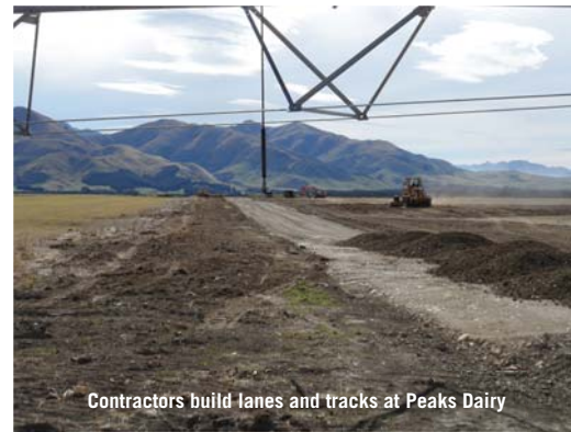
The site of the new 54 bale rotary cowshed at Peaks Dairy Ltd
